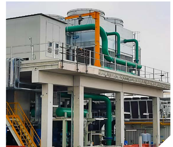
Construction site for Combined Heating and Cooling Power System in Barge Italy
